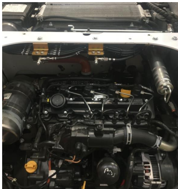
Figure 15 Pump Installed in Skid Steer Engine Compartment
